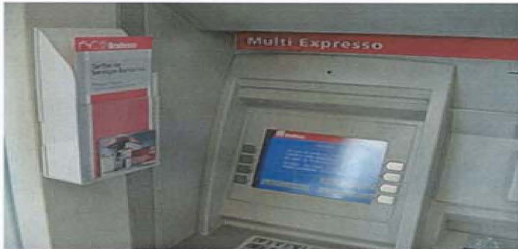
The camera shown installed and ready to capture PINs by looking down on the keypad as you enter your PIN.
